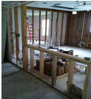
Kitchen before rehab
